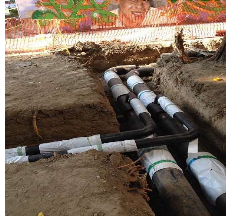
Zagreb's district heating network will undergo a major refurbishment and upgrade in the 2020 – 2023 period.
