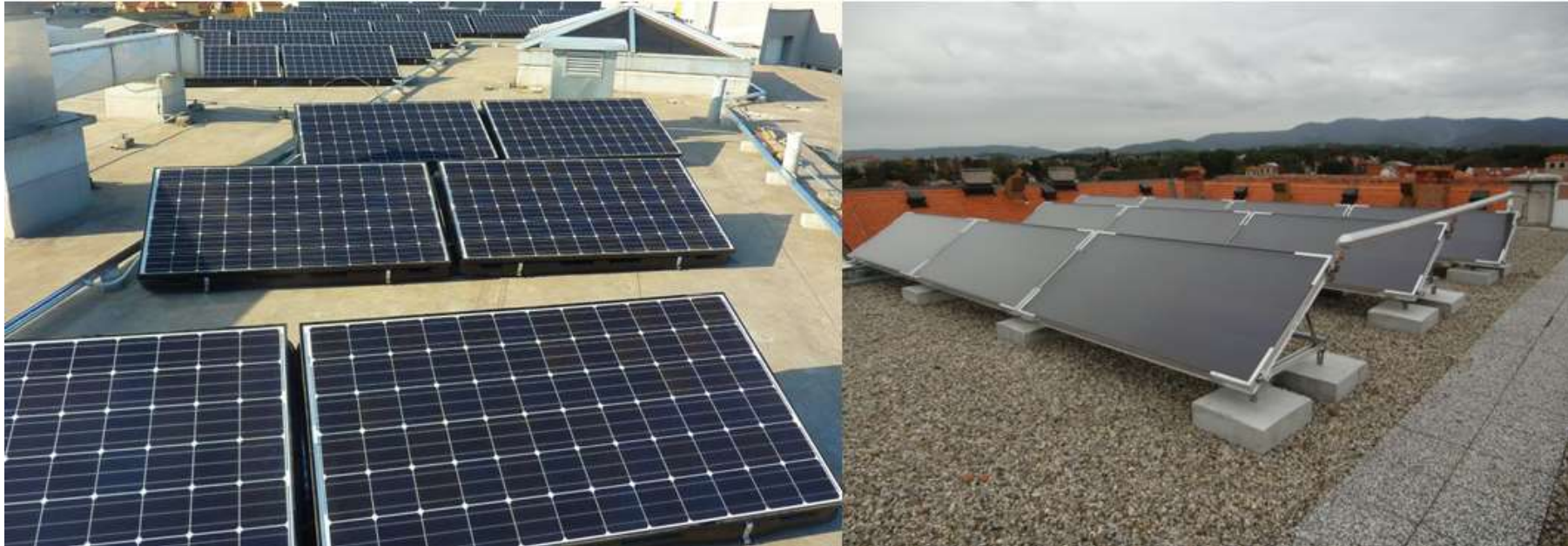
Photovoltaic & solar thermal collectors installed on public buildings
